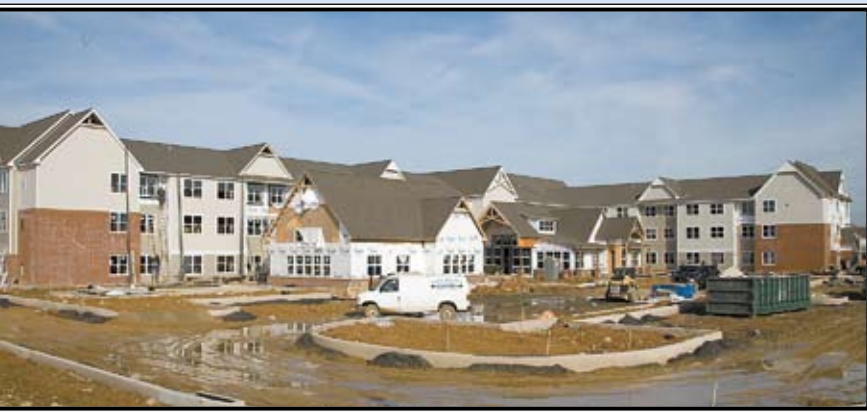
Less than a year after groundbreaking ceremonies were held, top, construction of the new 92-room Residence Inn nears completion.
