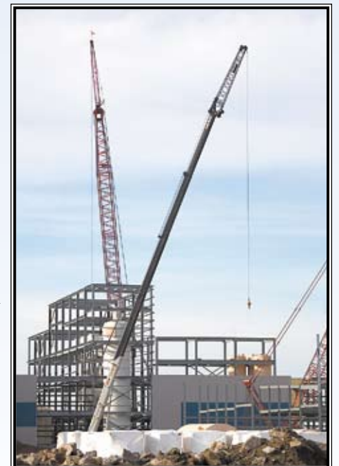
ADM's 500,000-square foot cocoa processing facility in Humboldt North is under construction.
